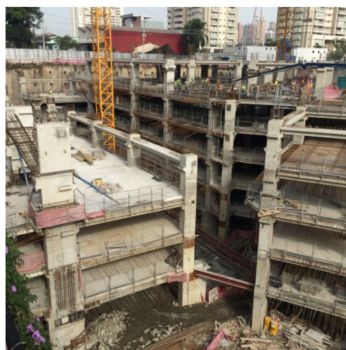
Figure 10. Lateral view of the mall during concrete phase of the fifth basement.
